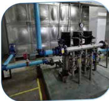
Water pipe network monitoring
