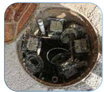
Urban domestic sewage monitoring
