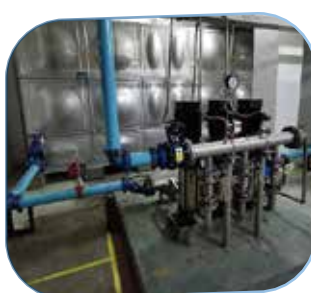
Water pipe network monitoring
