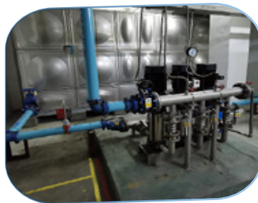
Secondary water supply
