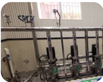
Municipal Pipe Network, Waterwork
