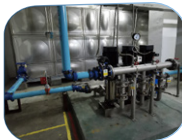
Secondary water supply
